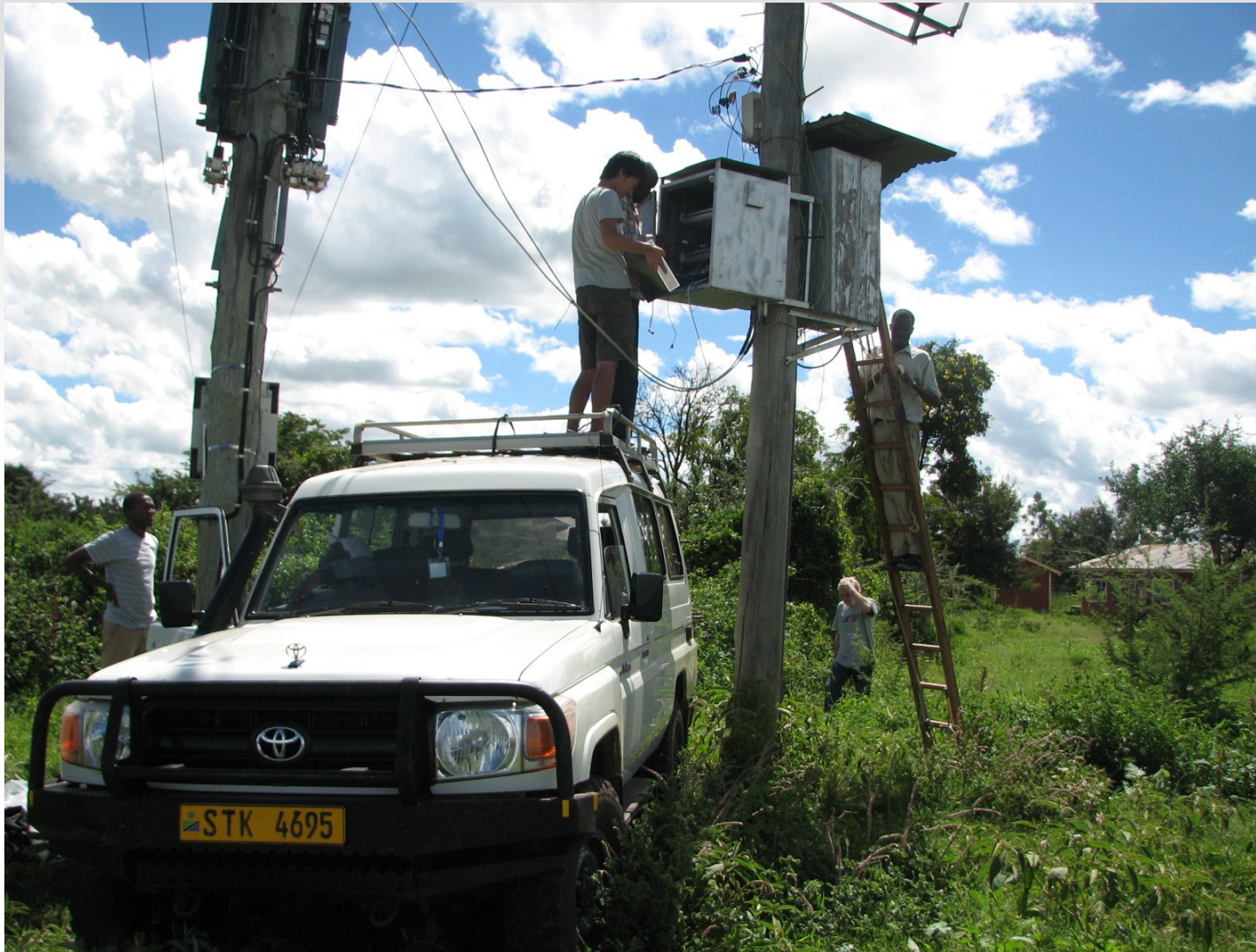
Router upgrade in Nata/Serengit spring 2012
